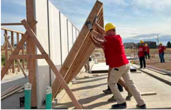
Volunteers raising a wall at the last two homes on Margaret Street in Deer Park during Veterans Build in September.
